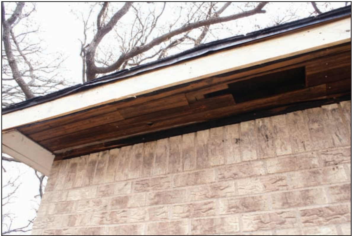
The homeowner witnessed embers blowing under the eaves and flames climbing the side of the house. Hours were spent putting out spot fires in the attic in order to save the house.
