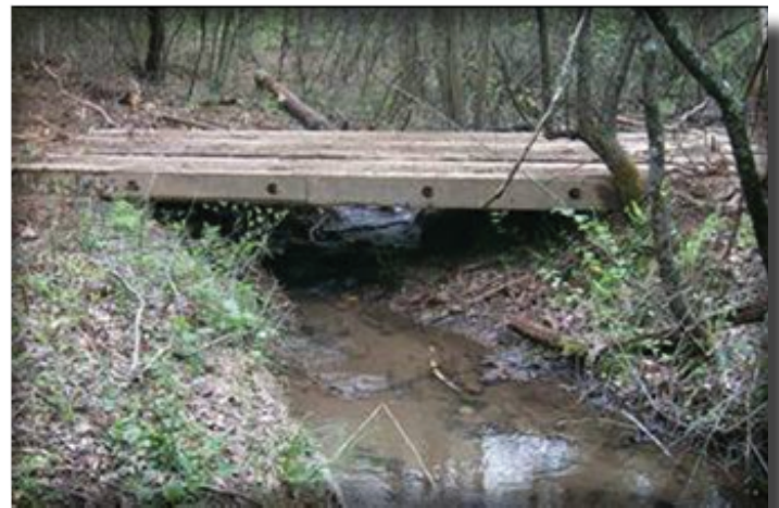
Bridgemats provide a good alternative for temporary stream crossings with minimal impacts to water quality.
