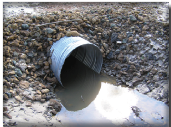
Culvert crossings should be properly sized and armored to prevent them from washing out.
